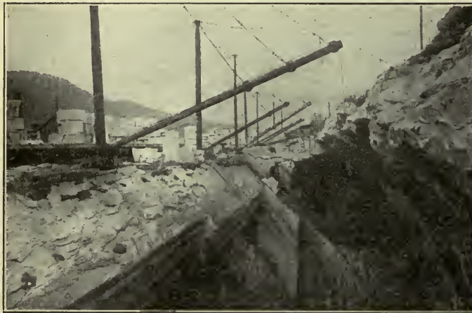
FIG. 160.—One of the marble quarries near Rutland, Vt. The stone is quarried out in the deep pit on the right, and the blocks are hoisted to the surface by the derricks.
